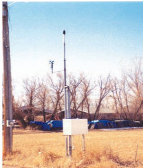
Remote Monitoring Terminal (RMT) with a weather collecting station.
