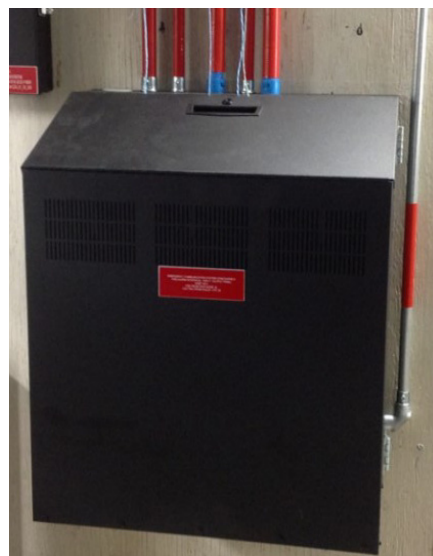
Figure 4-10: Fire Alarm/ECS Interface Cabinet
